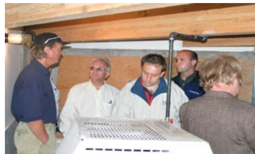
Contractor Leif Juell (Left) talks to Plug Power senior board member, John Elter (center), about a future fuel cell upgrade.
